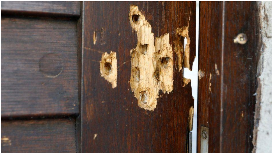
Figure 31 – Damages inflicted on the security door by the attacker's gunfire
