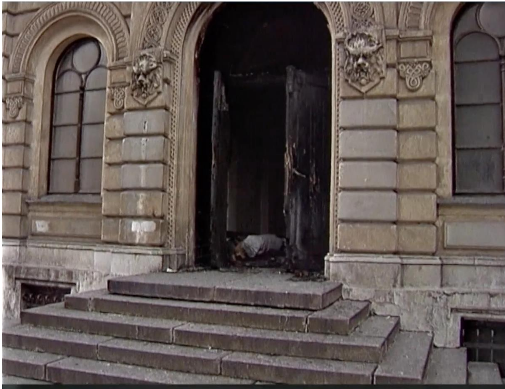
Figure 24 – Damage of the entrance door of the synagogue 132
