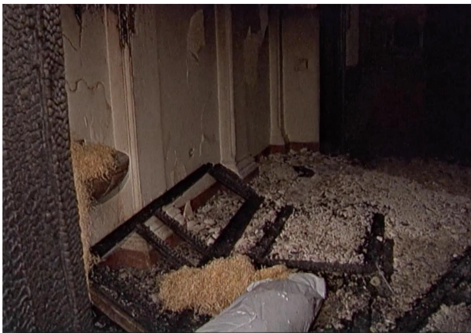
Figure 25 – Damage of the interior door, carpets and vestibule of the synagogue 133
