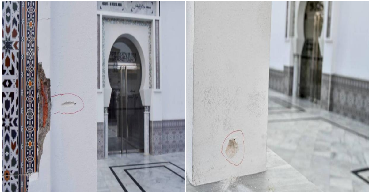
Figure 47 – The damage caused in the entrance of the Muley el Mehdi Mosque in Ceuta by the shootings 193
